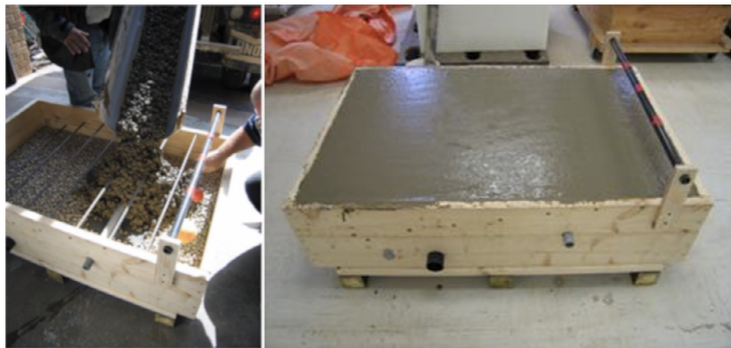
Fig. 9. Real data – case 2: Construction of the concrete box with seven 10-mm reinforcing bars at depths ranging from 0.5 to 15 cm. (Photos courtesy of Sensors & Software Inc.)
